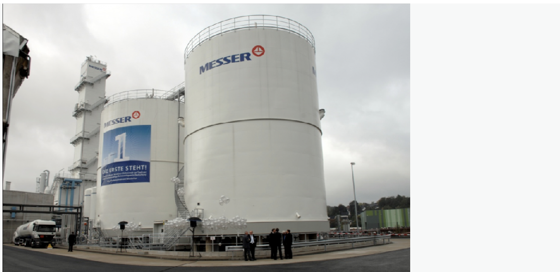
Figure 5: Air separation plant at Siegen, Germany. Source: Messer Industriegase GmbH
