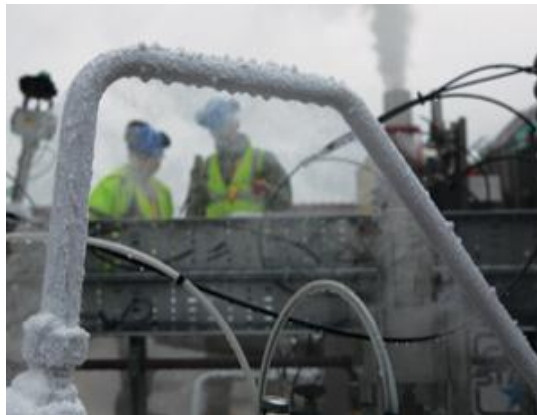
Excess energy from the power station is used to power a giant fridge ( Image: Jez Coulson/Highview )
