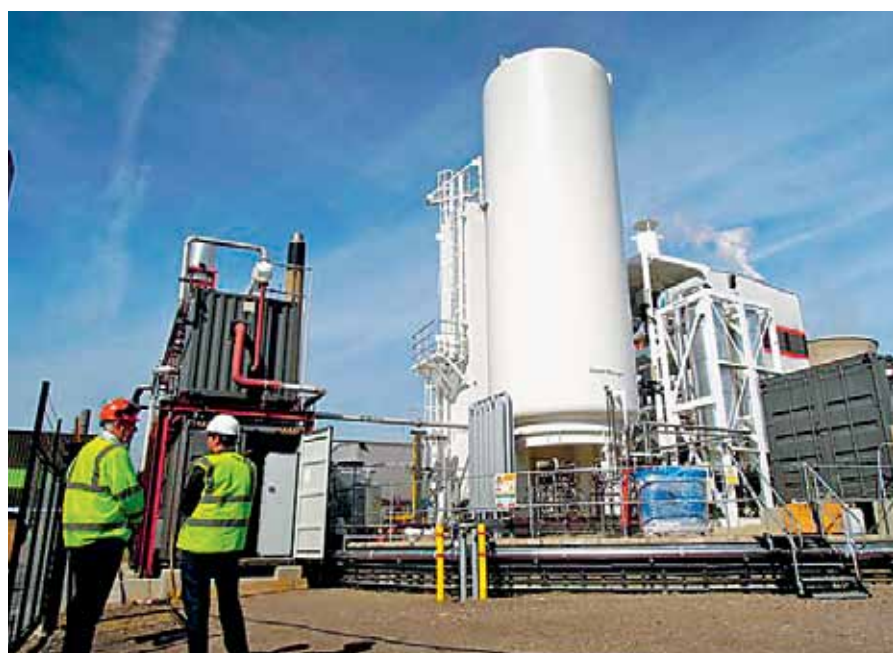
Cryogenic on-grid energy storage 2.5MW demonstration plant in Slough, UK.
